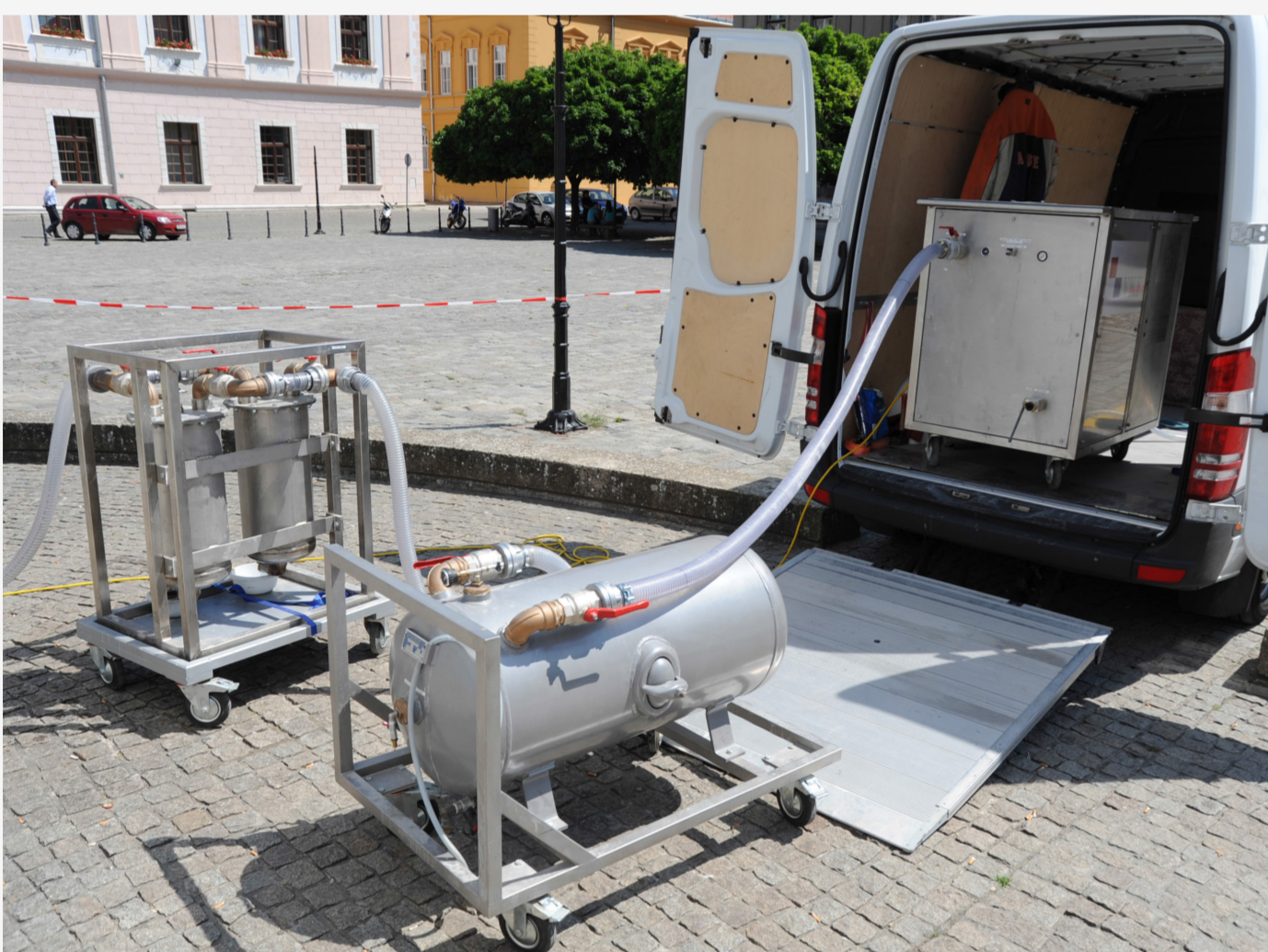
Figure 1: Mobile VCP equipment, vacuum pump (in truck), balance tank (middle), tank A&B combination (left; see Figure 2 for details).
