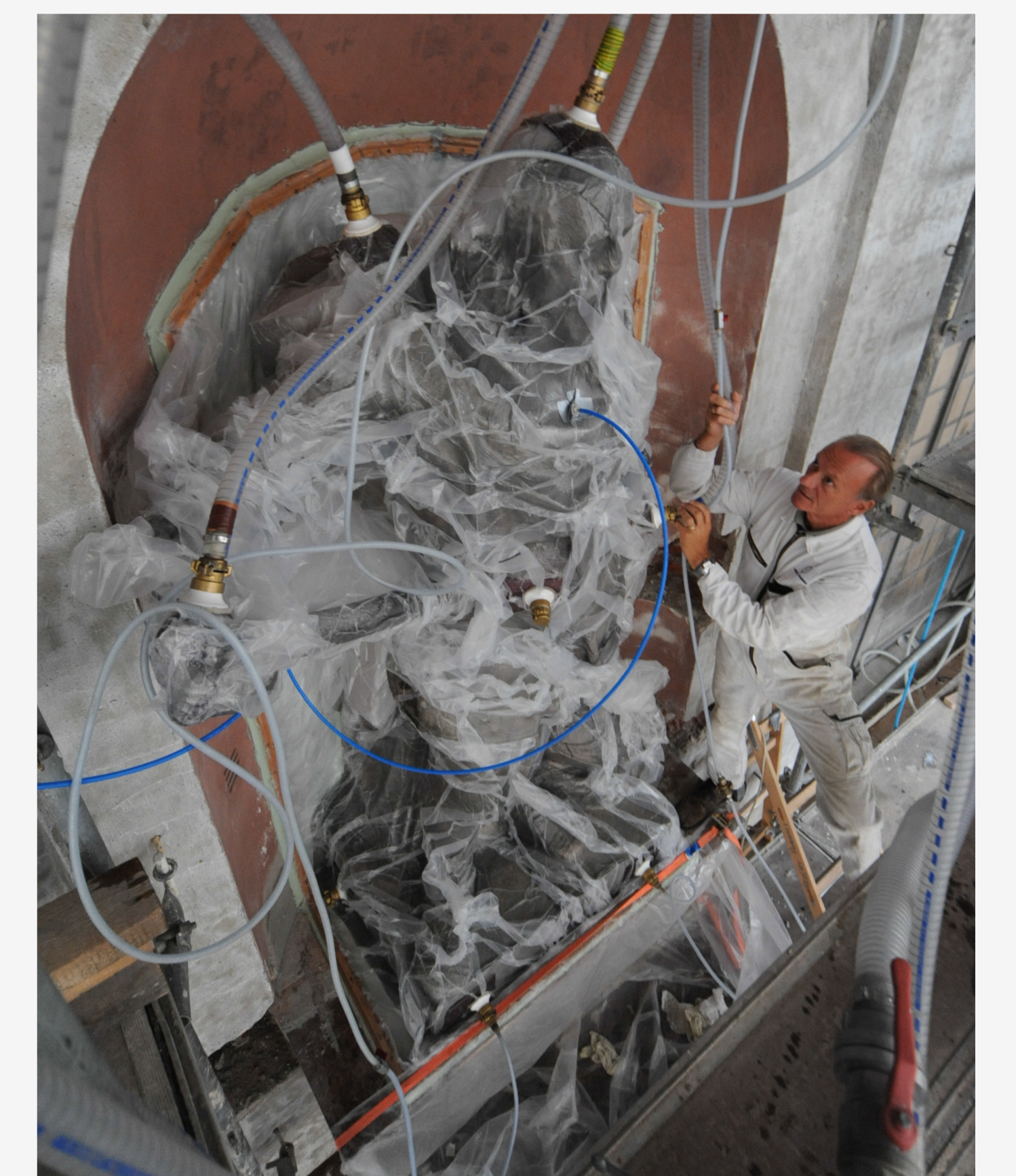
Figure 10: VCP conservation in situ of Duke Albrecht V., duration of treatment: 10 hours. Absorption of ESE: 50 kg.
