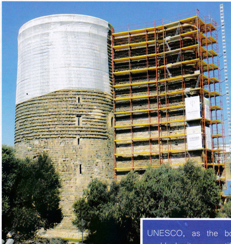
The bastion of the Maiden Tower, covered in scaffolding, with the upper part of the round tower shrouded in netting. This forced the swifts to start to occupy the nesting boxes, thereby enabling work on the façade of the tower. Photo: Erich Pummer.
