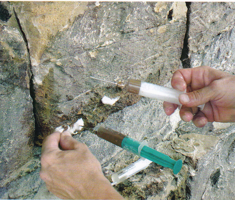
The damaged surfaces and structures are conserved stone by stone. Lime suspension and silicic acid ester are injected to fill the cracks and cavities. Photo: Erich Pummer.
